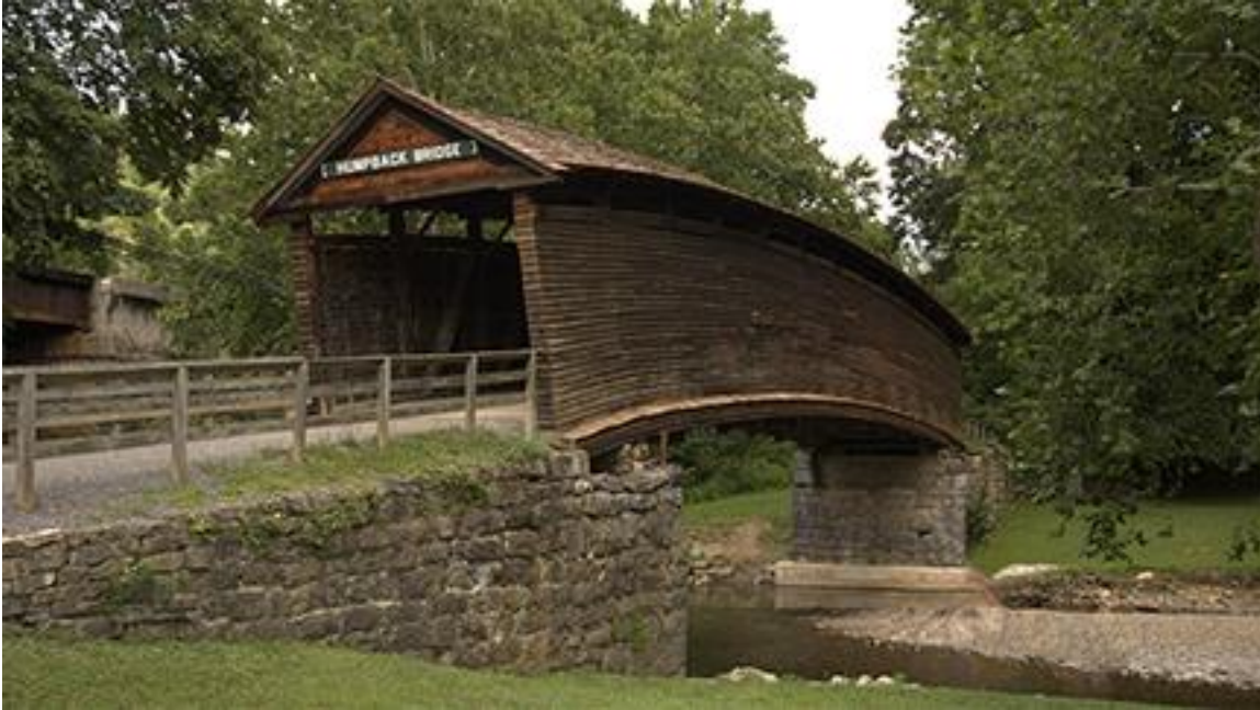
Figure 2. Stone Masonry Abutments and Stone Masonry Approaches on Humpback Bridge, 1857 (Alleghany County Structure No. 9007)
