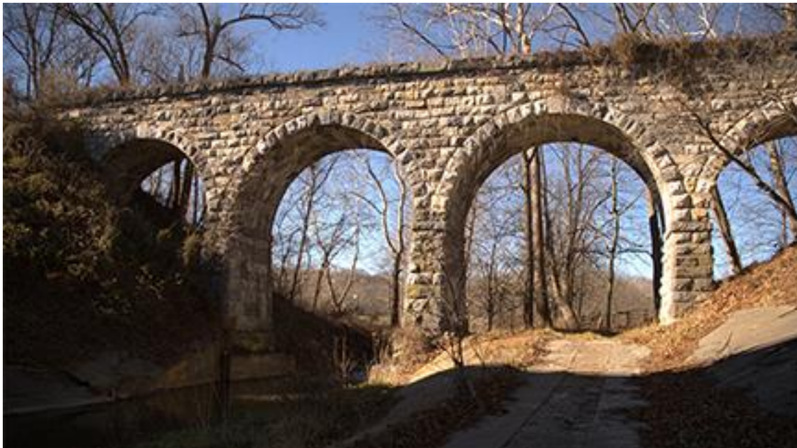
Figure 3. Stone Masonry Arch, Built as a Railroad Bridge, 1874 (Augusta County Structure No. 6997)
