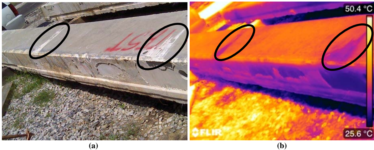
Figure 20. Comparison of (a) Digital Camera and (b) Infrared Camera Images of Bottom of Beam From Qualla Road Bridge. Note the encircled residue-covered locations.
