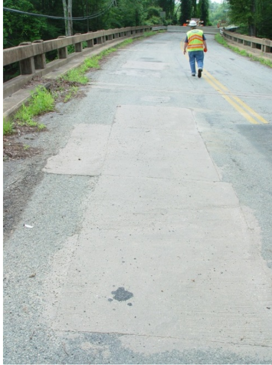
Figure 24. View of Adkins Road Bridge Deck. Vegetation is growing along the scuppers on both sides of the structure.
