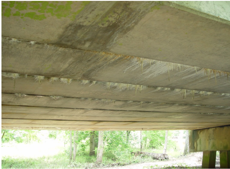
Figure 26. Efflorescence at Underside of Beam Joints of Adkins Road Bridge
