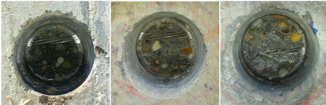
Figure 22. Condition of Prestressing Strands Through Concrete Coring of Qualla Road Bridge
