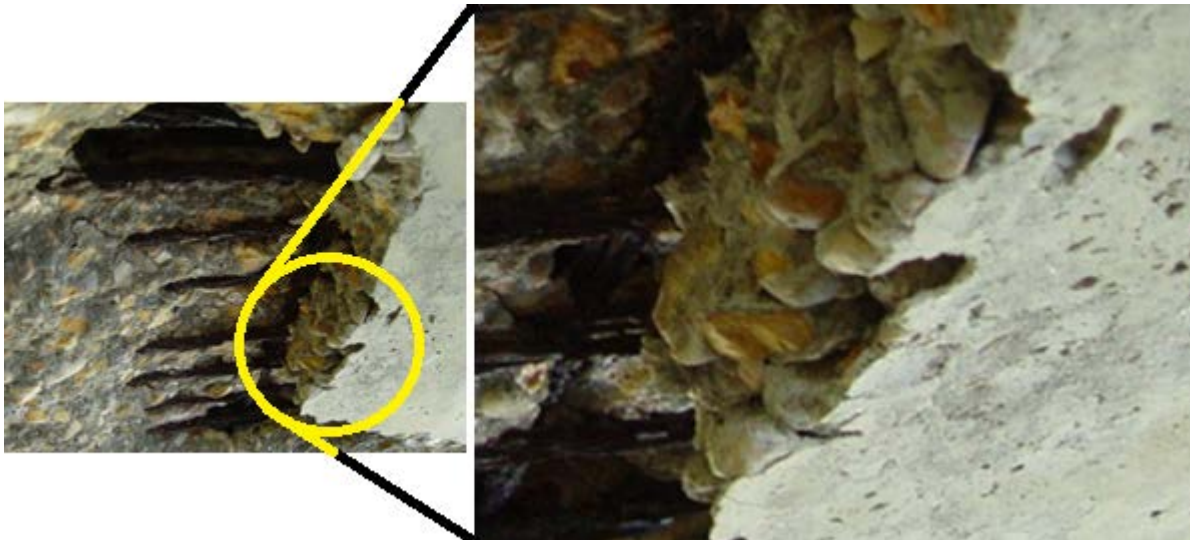
Figure 41. Adkins Road Bridge: Poorly Consolidated Concrete Below Broken Strands Near Quarter-Point Closest to Bent 3 in Beam 4, Span 3
