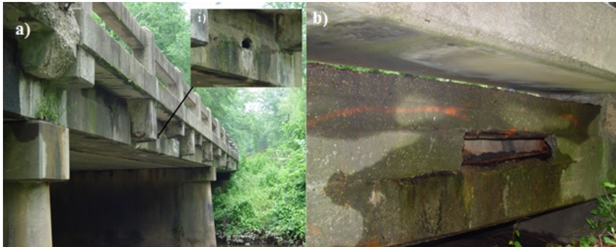
Figure 11. Qualla Road Bridge: (a) Side View With Magnified View of Hole and Efflorescence (Beam 9B), and (b) Hole on Exterior Beam (Beam 1A)
