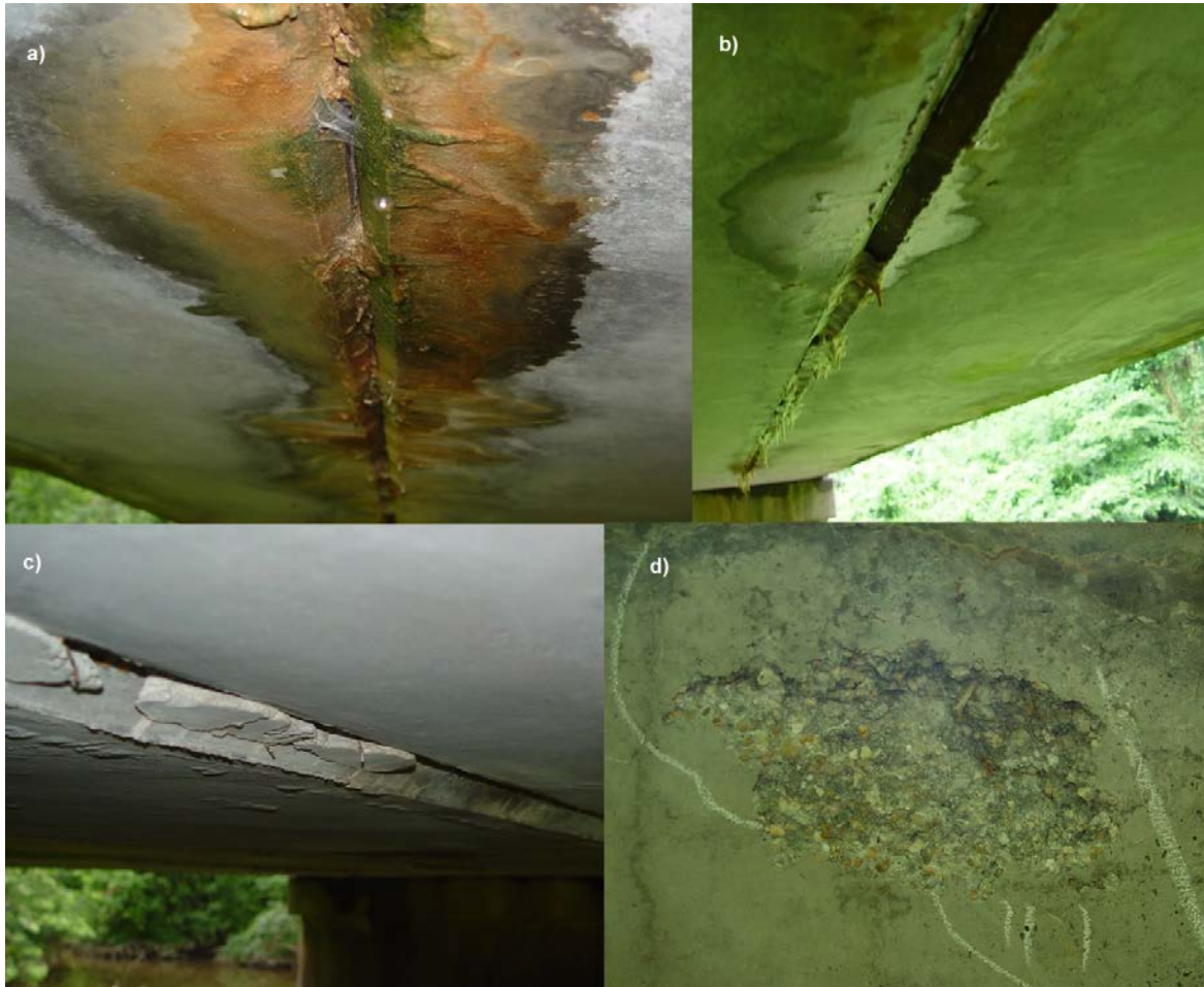
Figure 14. Visual Survey of Deck Underside of Qualla Road Bridge: (a) Moisture From Recent Precipitation; (b) Salt Stalactites; (c) Failure of Longitudinal Shear Concrete Joints Indicating Differential Movement Between Adjacent Beams; and (d) Shallow Spall in Soffit
