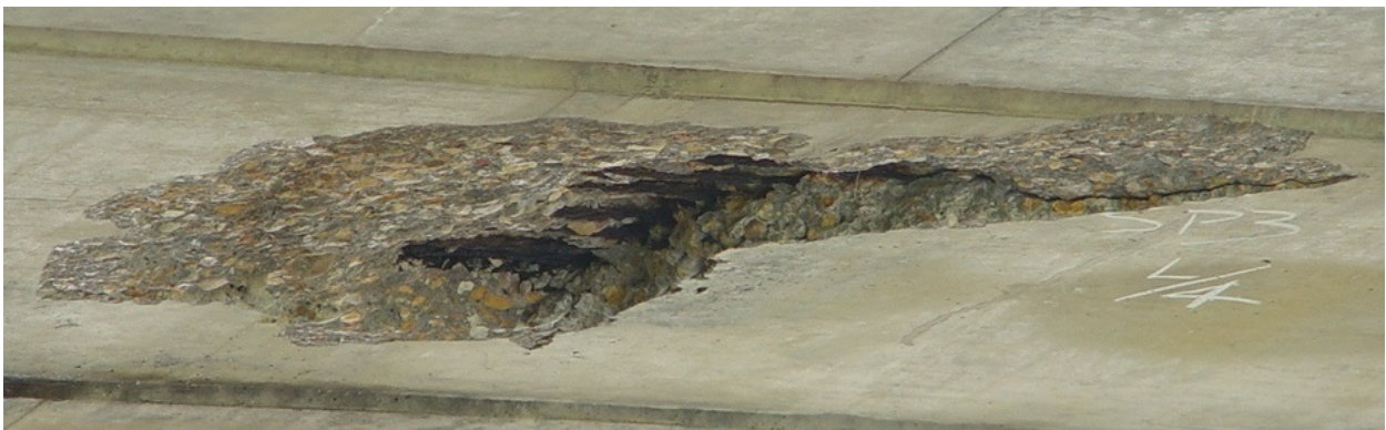
Figure 8. Spalled Concrete and Corroded Prestressing Strands in Beam 4 of Span 3, Near the Quarter-Point Closest to Bent 3, of Adkins Road Bridge
