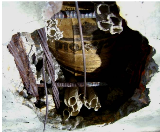
Figure 42. Adkins Road Bridge: Poorly Consolidated Concrete Near Quarter-Point Closest to Bent 2 in Beam 3, Span 3
