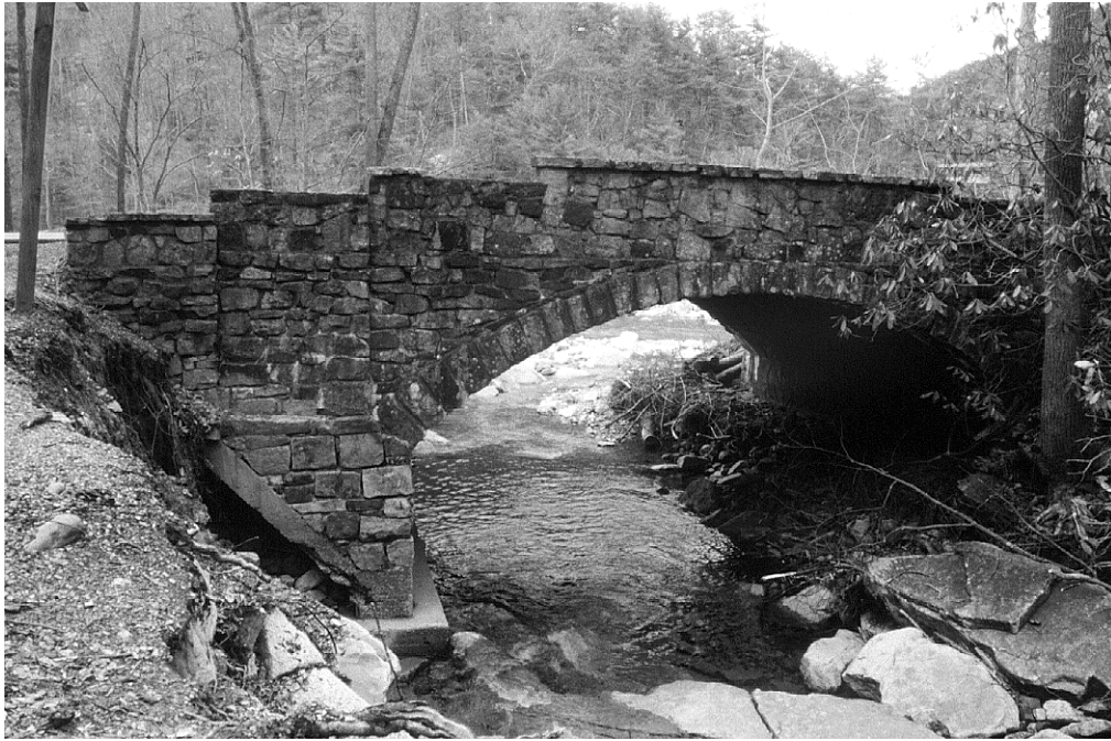
Figure 22. Rigid Frame with Stone Veneer, Built in 1940 as Part of the Improvements to Rt. 39 in Goshen Pass (Rockbridge County Structure No. 1012)
