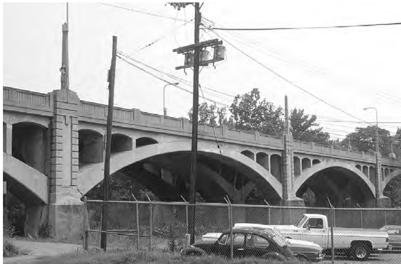
Figure 14. Open Spandrel Rib Arch with Art Deco Design Motifs, Built in 1926 (City of Roanoke Structure No. 1826)
