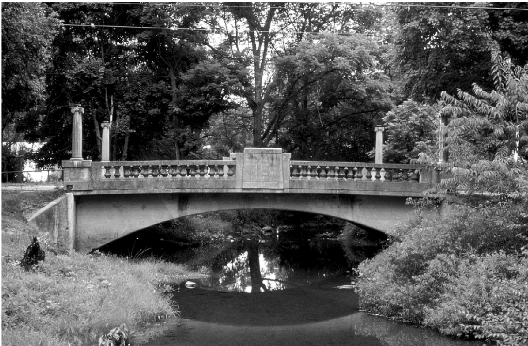
Figure 13. One of Lutten's Spandrel Braced Arches, with Decorative Concrete Elements and "Park Rail," Built in 1929 (Bland County Structure No. 1021)
