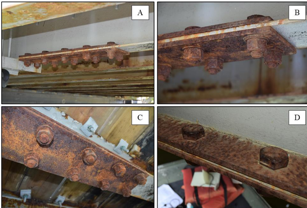
Figure 32. Photographs of Bolted Repair Type 3 Made of Weathering Steel Plate and Fastener Assemblies on the Onancock Bridge: (A) general view; (B) side view close-up; (C) view of bottom of bottom flange; (D) view of top of bottom flange.
