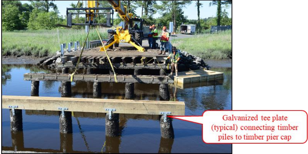
Figure 15. Photograph Showing Galvanized Tee Plates Connecting Timber Piles to Timber Pier Cap
