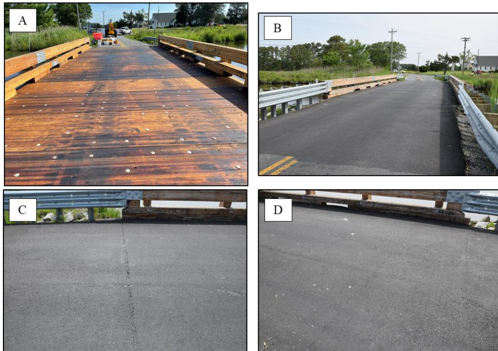
Figure 17. Photographs of the 2022 Holdens Creek Bridge Deck: (A) before asphalt overlay; (B) after asphalt overlay; (c) view of asphalt reflective cracking at north abutment; (D) view of asphalt reflective cracking at south abutment.
