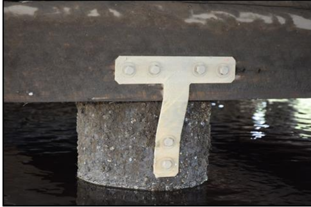
Figure 24. Photograph of Galvanized Tee Plate Connection Between Piles and Pile Cap on the 2022 Holds Creek Bridge
