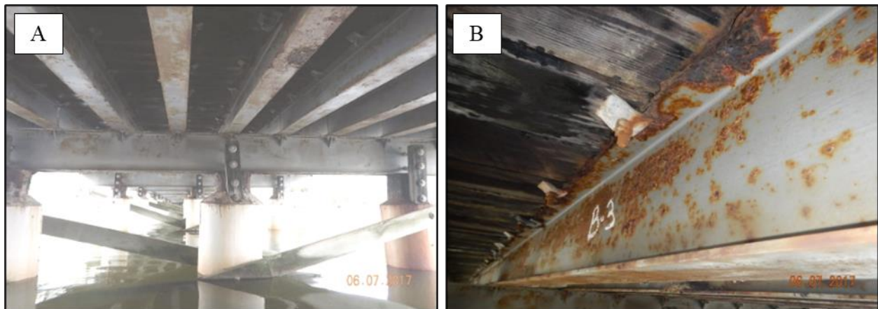
Figure 26. Photographs Showing Coating on Beams of the Onancock Bridge in 2017: (A) loss of coating and surface rusting along beams; (B) section loss on top flange of beams.
