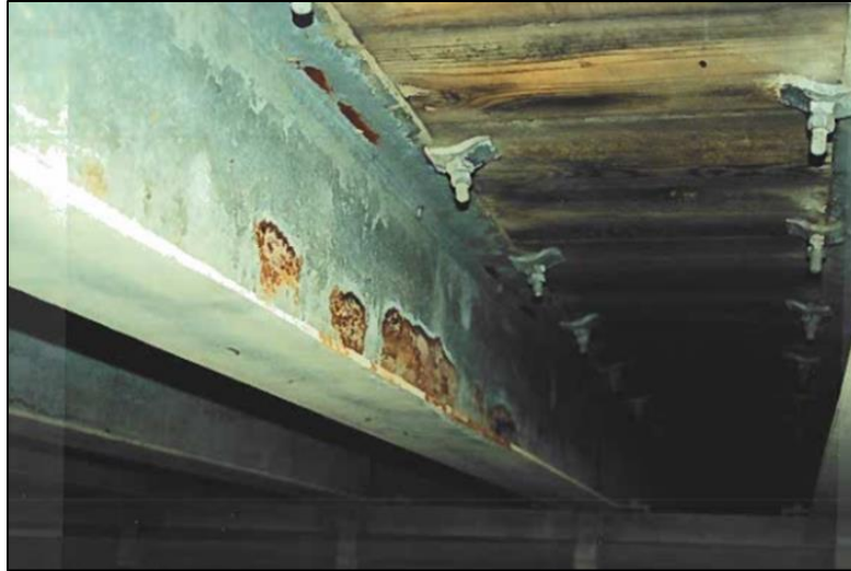
Figure 5. Photograph Showing Coating Breakdown for the 1993 Holdens Creek Bridge in 1999, Indicating Loss of Complete Coating Protection After 6 Years
