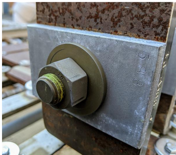
Figure 46. Photograph of Long-Term Corrosion Sample 16
