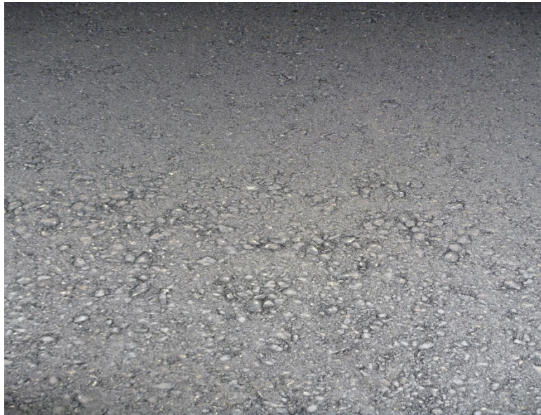
Figure 1. Example of Segregation Observed for 45% RAP Mixture. RAP = reclaimed asphalt pavement.
