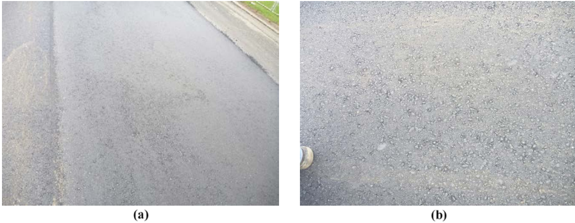
Figure 3. Example of Segregation Observed: (a) 30% RAP mixture; (b) 40% RAP mixture. RAP = reclaimed asphalt pavement.
