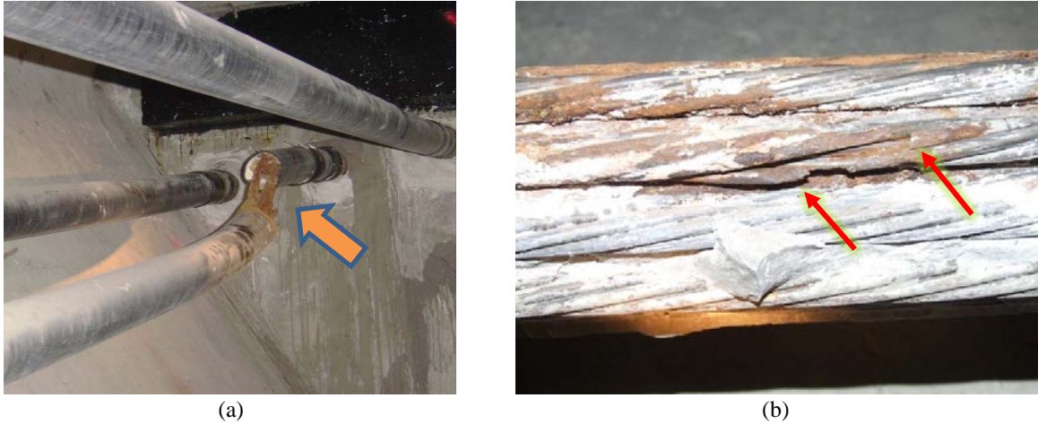
Figure 1. Corrosive Attack on Post-Tensioned Structural Strand: (a) corrosion of individual strand wires ultimately causing an overload failure of the middle external tendon (orange arrow); middle tendon is hanging by the broken wires inside the other half of the duct; (b) section loss in high-strength steel strand, with red arrows showing ends of a fractured wire
