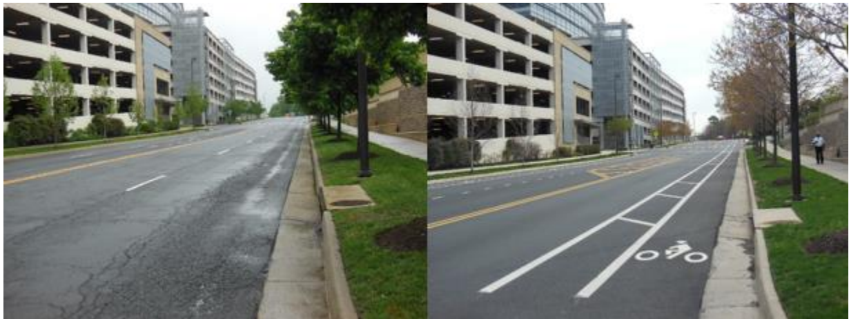
Figure 5. Before (Left) and After (Right) Photographs of Road Diet on Bluemont Way
