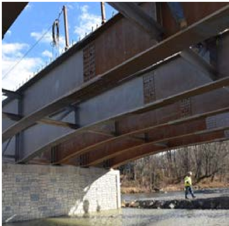
Figure 26. Various Stages of Patina on Steel Girders
