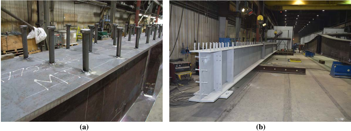
Figure 18. Carbon Steel Shear Studs: (a) top flange of beam; (b) top flange and web after mill scale removal
