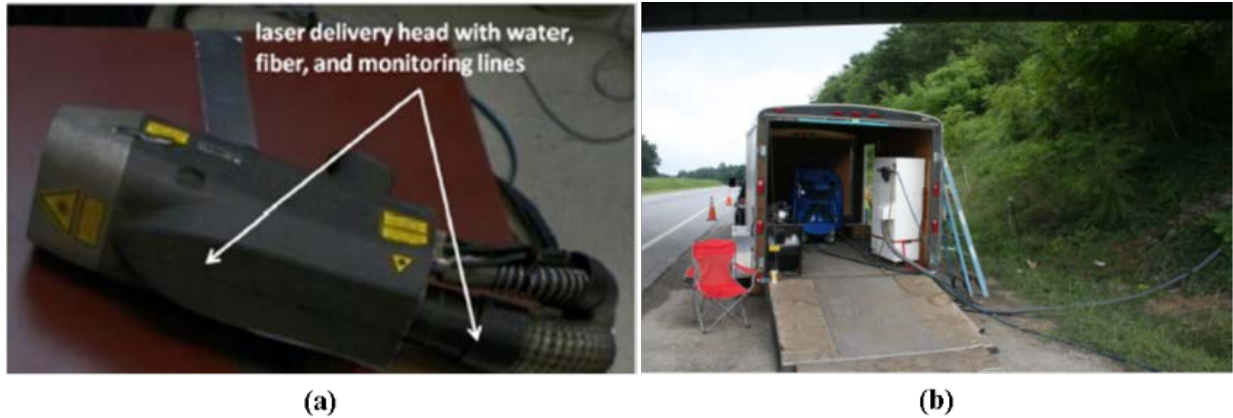
Figure 36. LACR System During Cleaning: (a) cables exiting back of laser optic; (b) portable generator and on-site cables. LACR = laser ablation coating removal.
