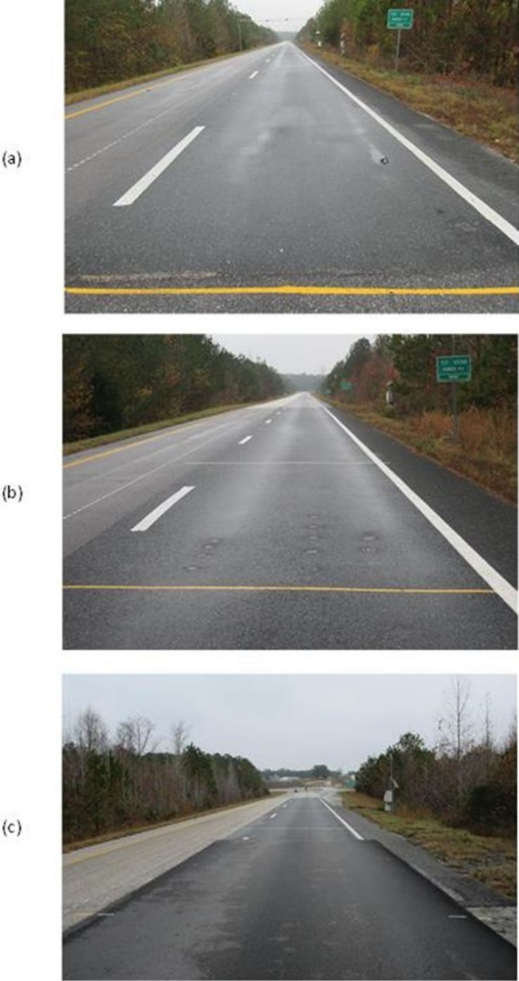
Figure 5. Visual Condition of VDOT Sections at NCAT Test Track: (a) Section N3; (b) Section N4; (c) Section S12.
