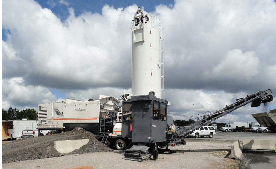
Figure 2. Cold Central Plant Recycling Plant
