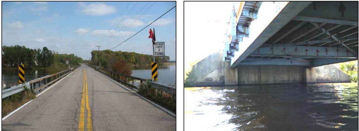
Figure 6. Original Bridge Over Swift Creek: left, 3 ton posting in spring 2010; right, underside of bridge
