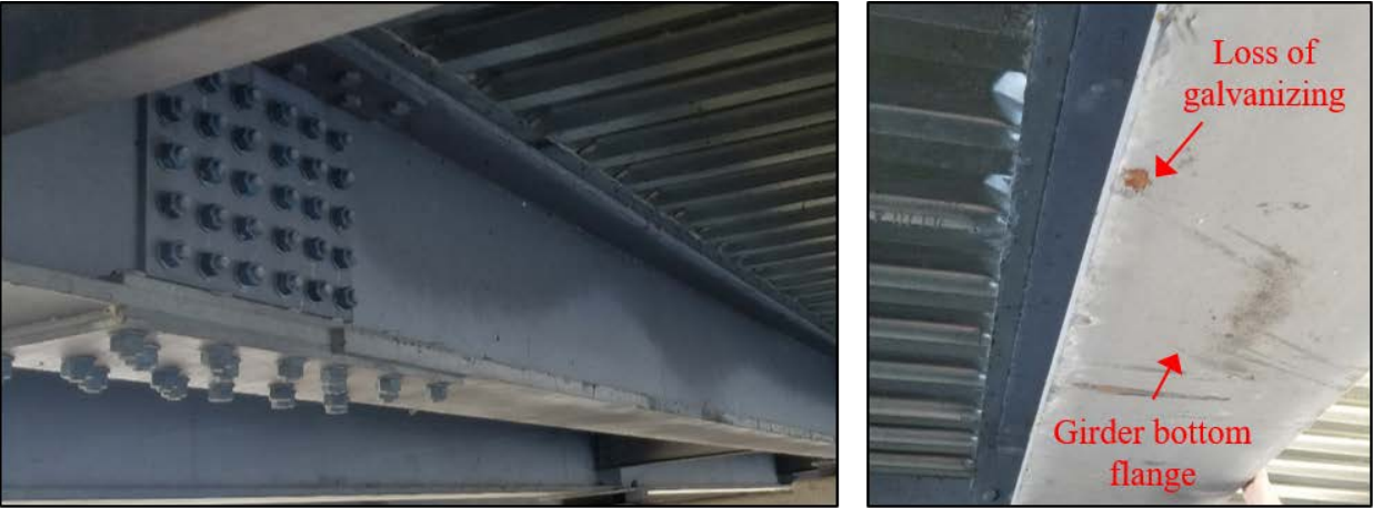
Figure 10. Visual Condition of Galvanized Weathering Steel Girder in March 2018: left, an example of the general condition; right, the only location exhibiting loss of galvanizing coating and showing the underlying weathering steel girder
