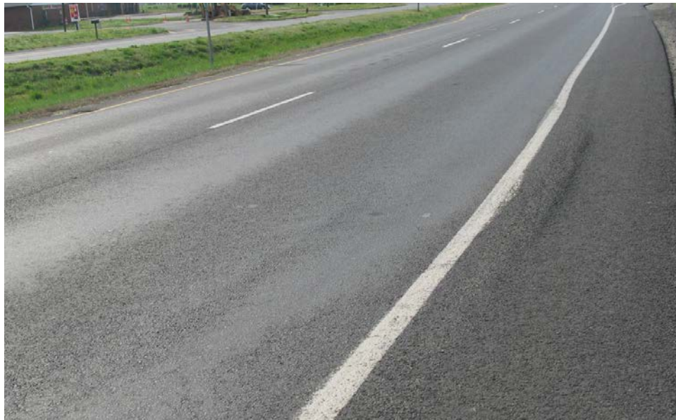
Figure 1. Flushing, Rutting, and Shoving in SMA-9.5 Pavement on US 17 Near Opal, Virginia. SMA = stone matrix asphalt. Source: McGhee et al. (2010).
