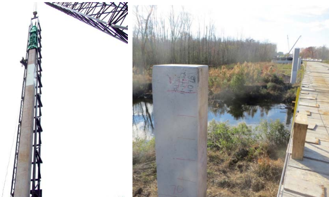
Figure 8. Preparing for Pile Driving (left); Pile in Place after Driving Showing No Signs of Damage to Upper Portion of Pile (right)
