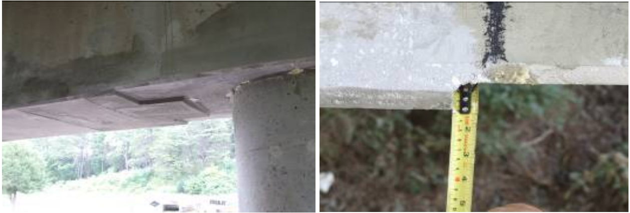
Figure 11. More Cover Depth in Repair Area of Route 712 Bridge Provided by Lowering of Formwork: Overview ( left ) and Measured Difference of Protrusion ( right )
