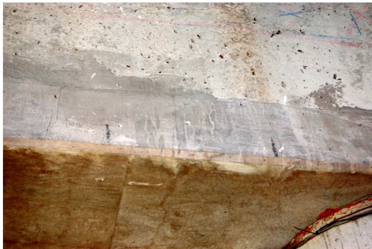
Figure 14. Tight Shrinkage Cracks in Repair Area of Route 712 Bridge in 2017
