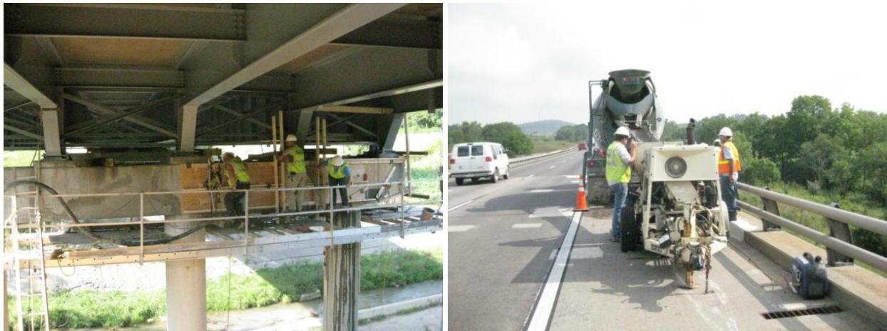
Figure 6. Deteriorated Pier of I-81 Bridge During Placement (left) and Small Pump on Deck (right)
