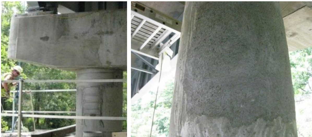
Figure 19. SCC With Smooth Surface (left) and Shotcrete Rough Surface (right) of Route 712 Bridge
