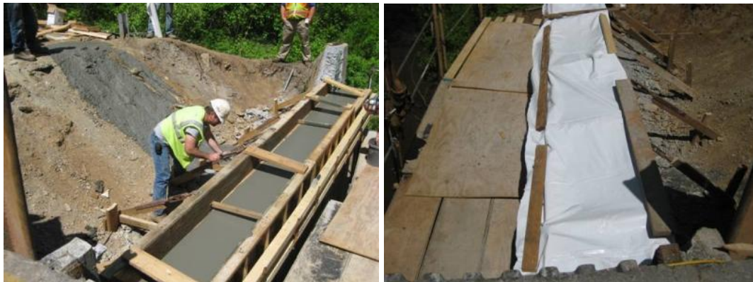
Figure 2. Concrete Finishing Before Curing (left) and Plastic Covering (right) for Route 699 Bridge
