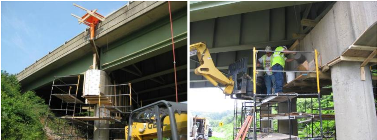
Figure 5. Funnel Being Used to Gain Pressure From Height Difference During Placement ( left ) and Manual Placement Method Using Container and Bucket ( right ) for Route 712 Bridge
