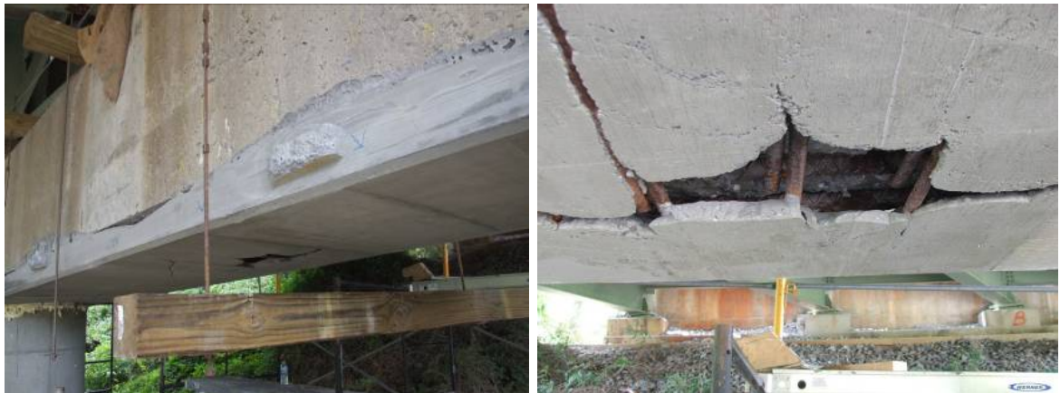
Figure 10. Ports Lower Than High Points (left) and Void at Bottom With Shy Cover (right) for Route 712 Bridge
