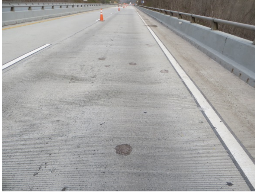
Figure 15. Small Dark Spots Attributable to Repair of Holes Left When Bag Pieces Were Removed From Bridge Deck
