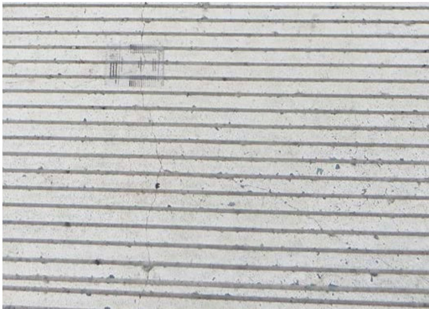
Figure 14. Plastic Shrinkage Cracking in RSLMC in Left Lane of Westbound Bridge. RSLMC = latex-modified concrete with Rapid Set cement.
