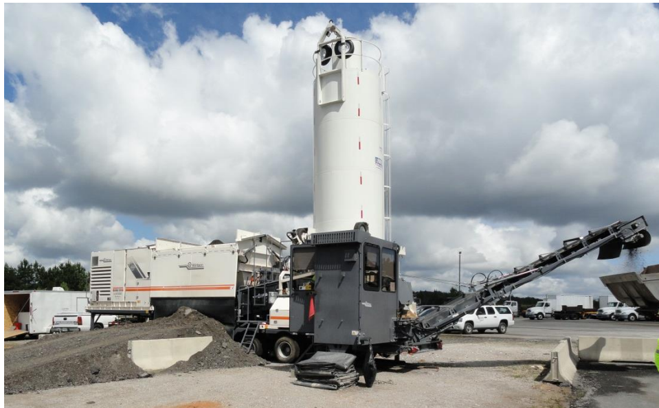
Figure 2. Cold Central Plant Recycling Plant at NCAT Test Track
