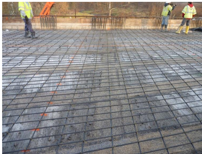
Figure 8. Box Beams and Reinforcement for Route 1421 Linville Creek
