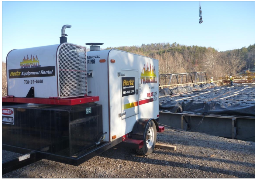
Figure 7. Heating System Used for Placements B, C, D, and E for Route 633 Covington
