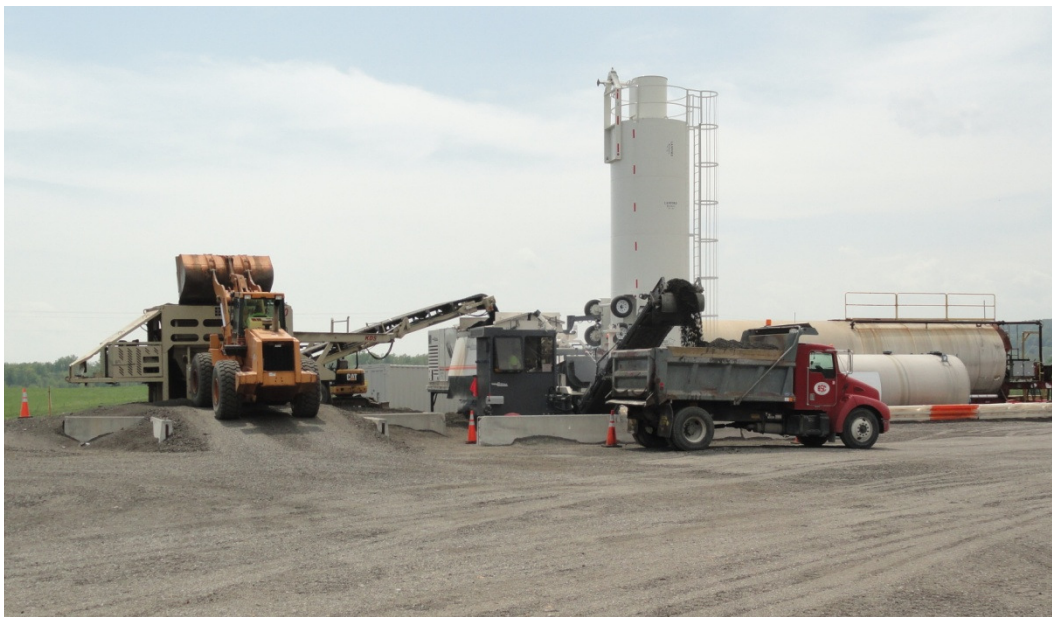
Figure 4. Cold Central-Plant Recycling Plant
