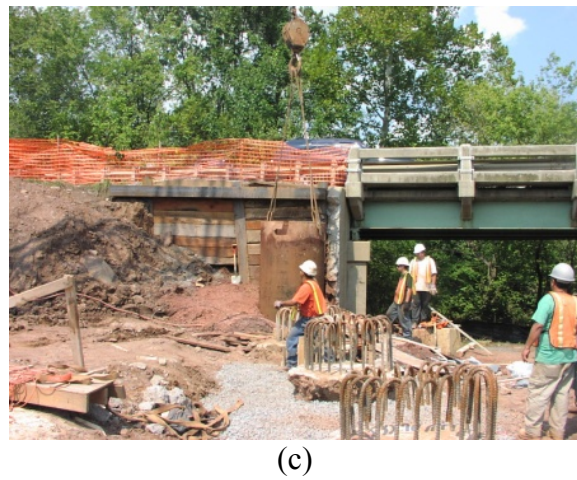
Figure 5. Placement of conventional concrete mixture in drilled shaft. (a) Concrete flows down the chute into shaft; (b) steel caisson is lifted slightly; and (c) then completely removed. Completed drilled shafts are visible in the forefront of Figure b and Figure c.
