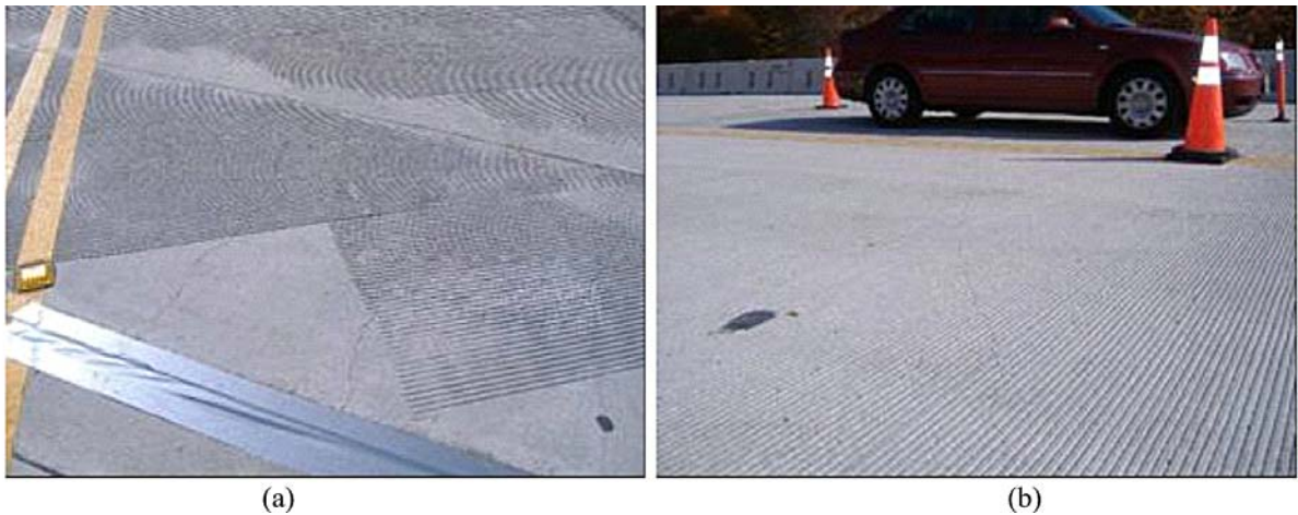
Figure 14. Cracks in Concrete on Stage I Southbound (ECR) Deck. (a) Cracks perpendicular to expansion joint, (b) Crack crosses diagonally across deck surface.
