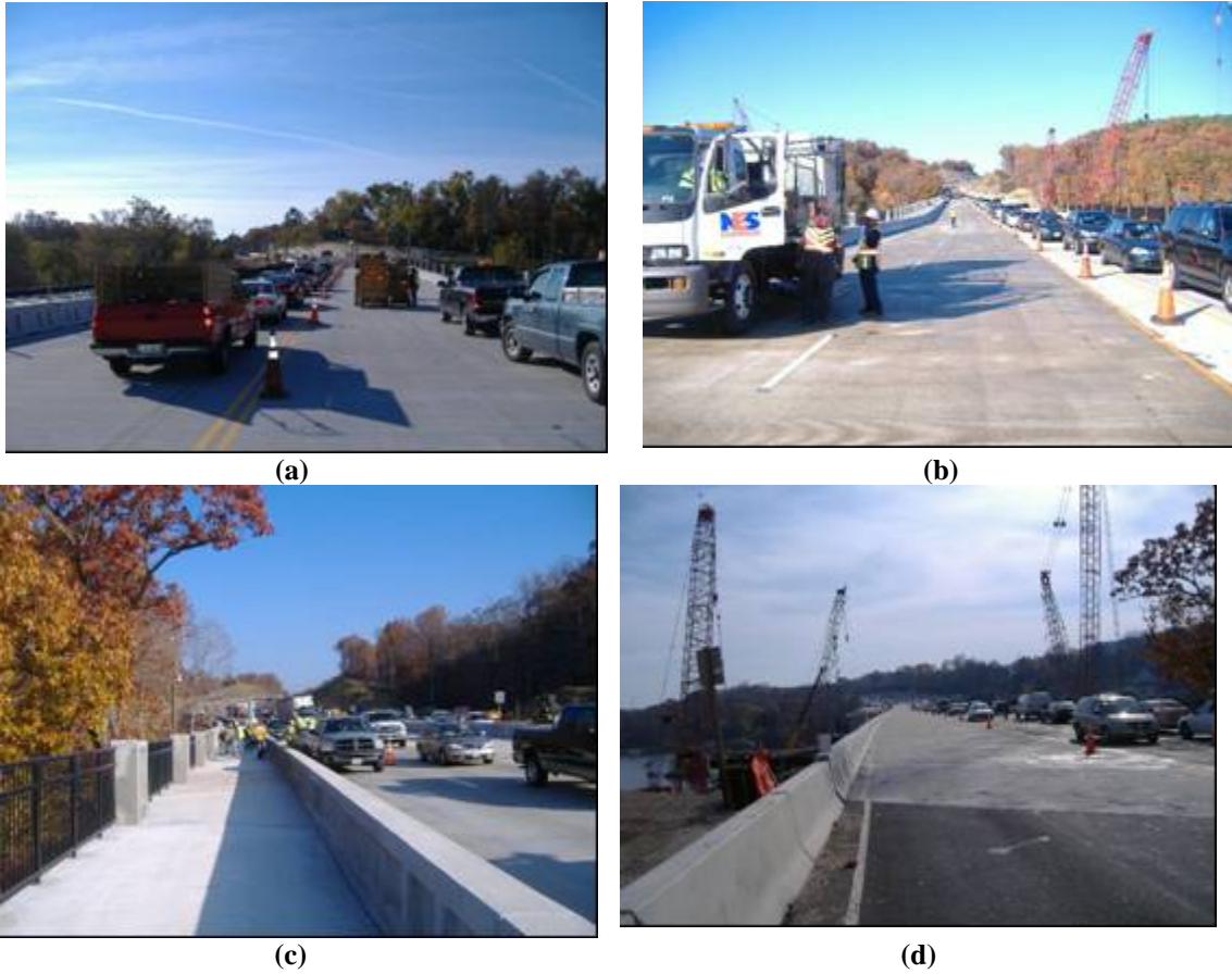
Figure 33. Traffic Configurations During Deck Sealing Operations. (a) Facing south, one lane open in each direction to left of median, (b) Facing north, one lane open in each direction, (c) Facing north, two southbound lanes and one northbound lane, (d) Facing south, one lane in each direction.
