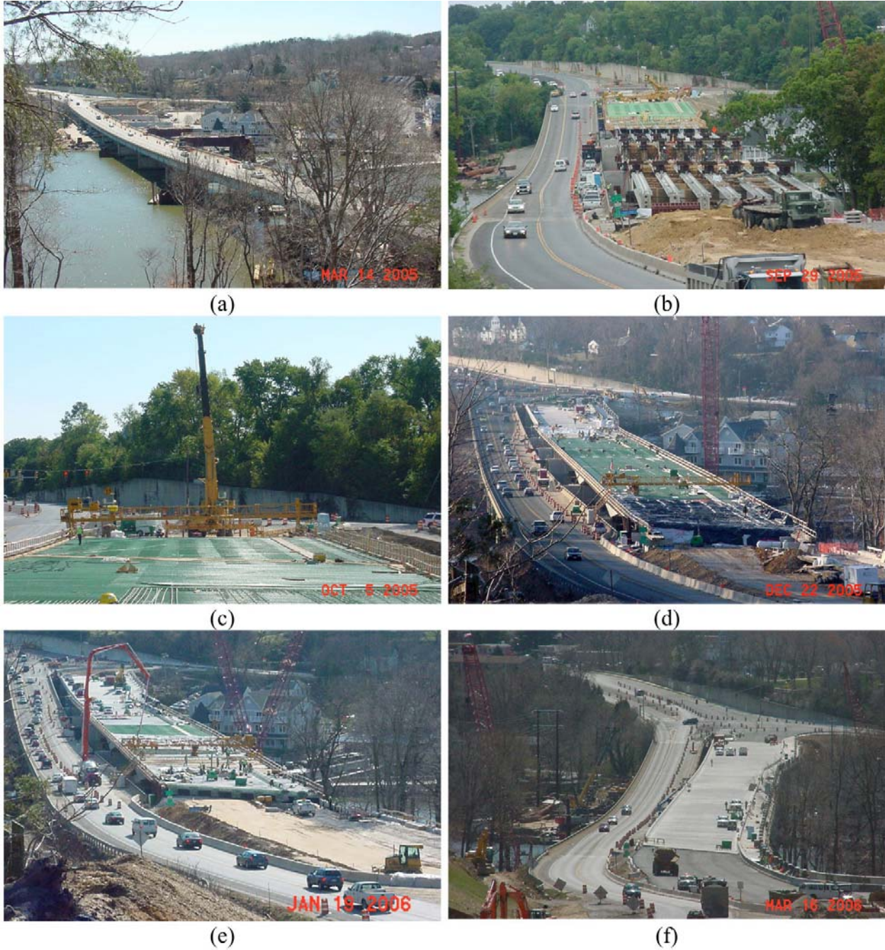
Figure 10. Construction of Southbound (ECR) Deck. (a) Substructure under construction, (b) ECR on southern end of deck, (c) Close-up of deck, (d) ECR placement near completion, (e) Placement of concrete in deck, (f) Concrete placement complete.
