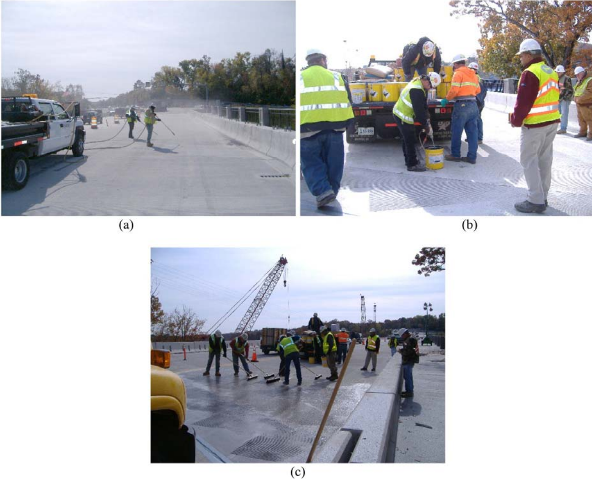
Figure 15. Crack Sealing of Southbound (ECR) Deck. (a) Cleaning of deck, (b) Mixing of epoxy, (c) Application of epoxy to deck surface.
