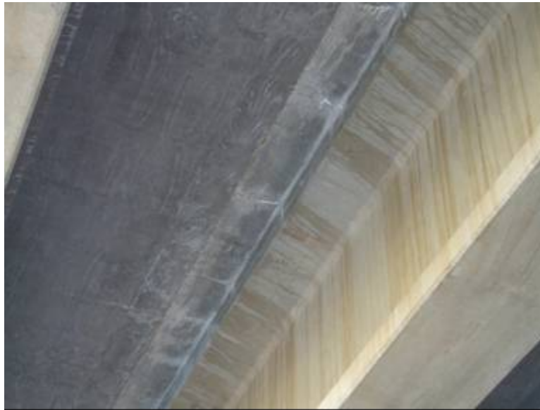
Figure 26. Short Efflorescence Pattern Adjacent to Girder on Underside of Southbound Deck
