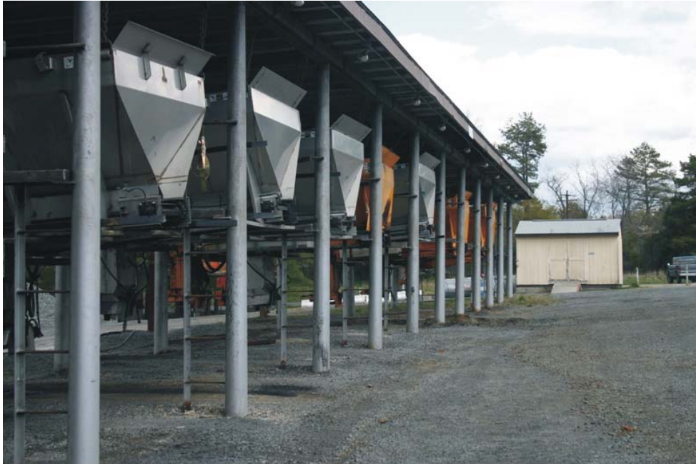
Figure 1. Salt-Spreader Racks Typical of Those Found at VDOT Area Headquarters Maintenance Facilities
