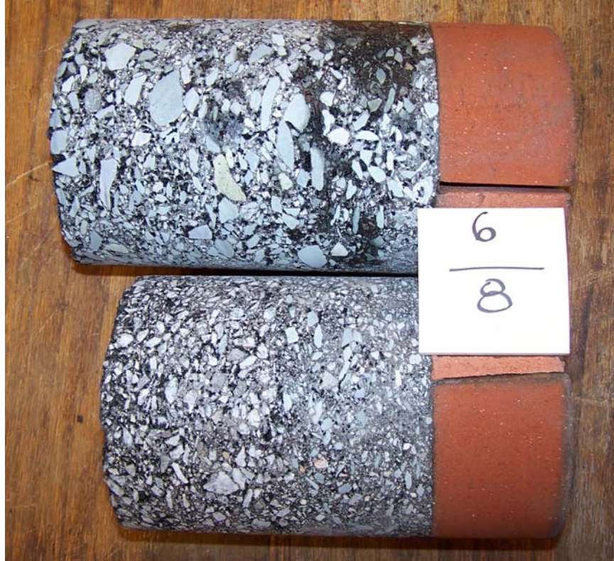
Figure B4. Example of Non-Uniformity in Particle Size Distribution and HMA Layer Thickness (specimens collected at intersection of 4th Street and Jefferson Street)
