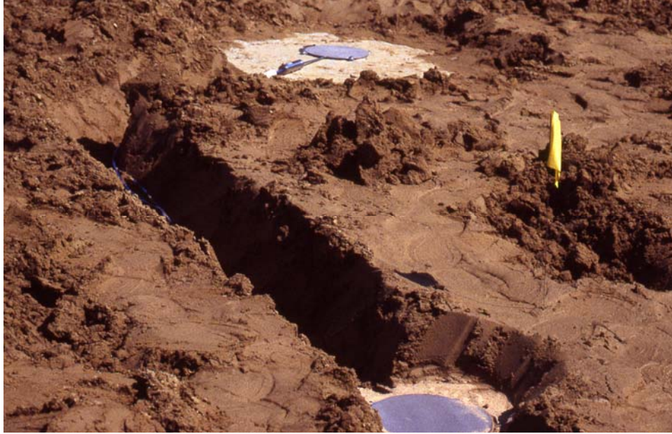
Figure 6. Pressure Cells 5 and 7 (Foreground)
