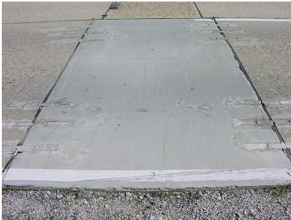
Figure 8. Discontinuous Joint at Dowel Retrofit
