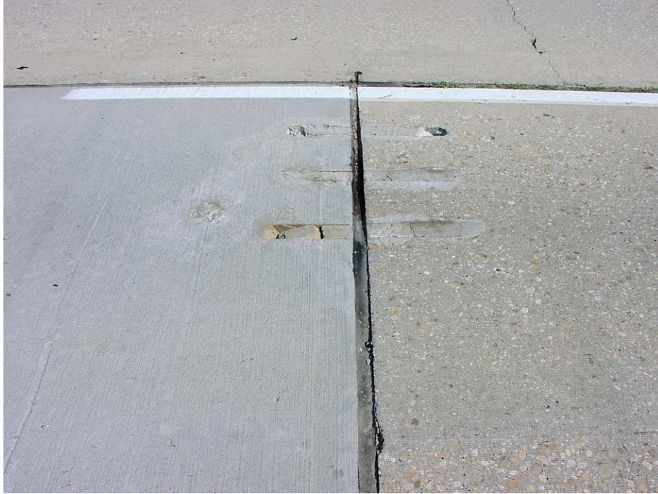
Figure 12. Missing Silicone Joint Sealer
