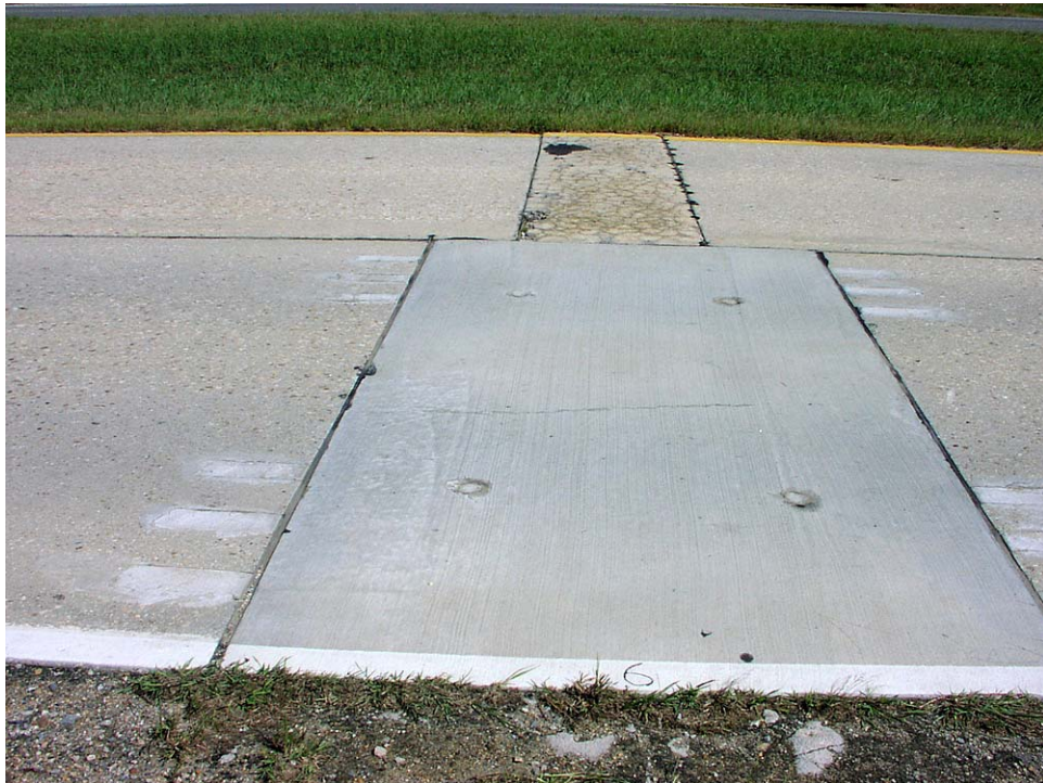
Figure 11. Crack Propagating Between Wheel Paths in Patch with Cast-In Dowel
