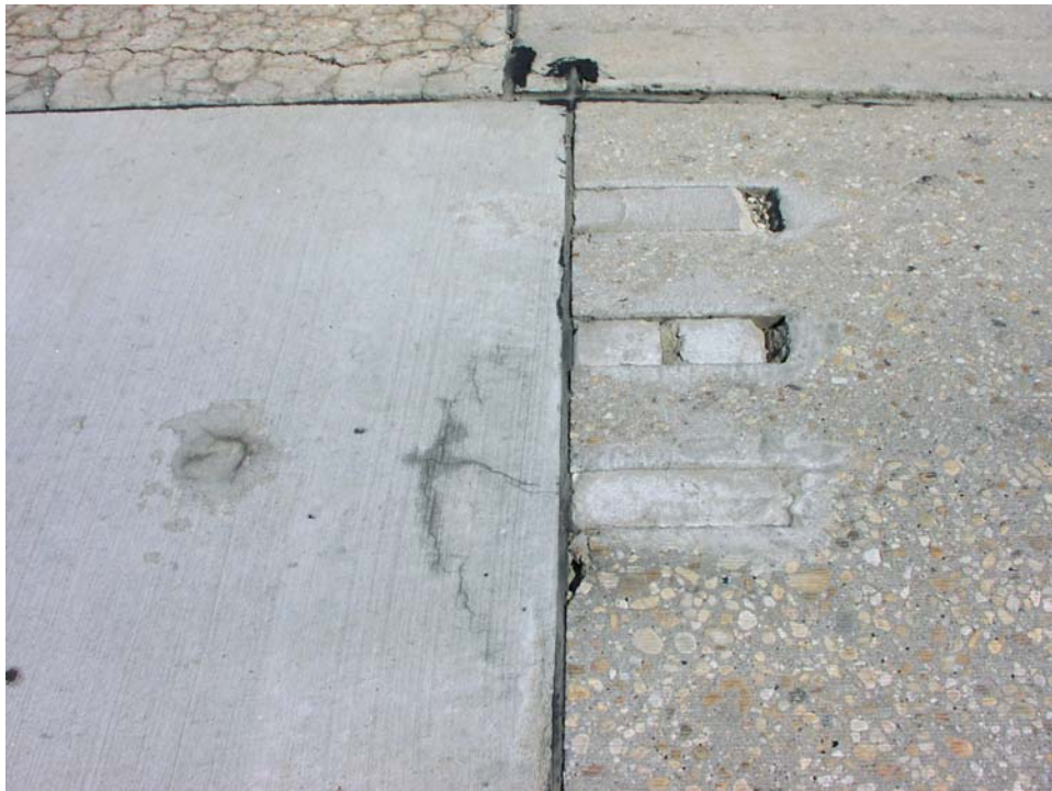
Figure 9. Cracks Propagating into Patch Cast With Dowel
