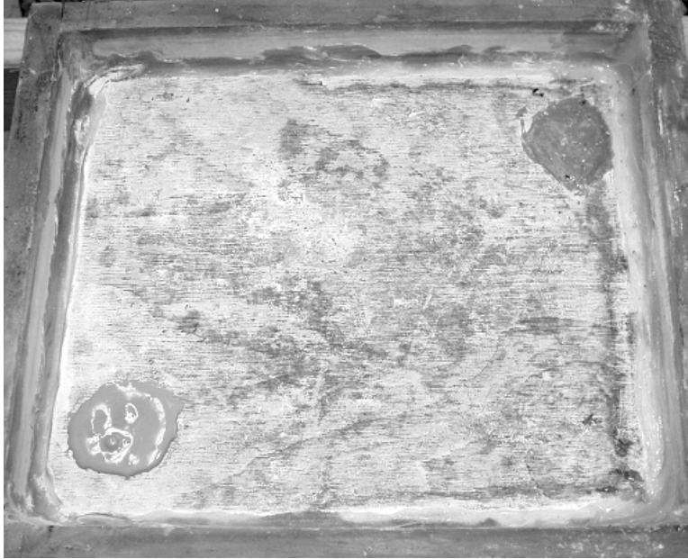
Figure 17. Concrete Surface Never Sandblasted
