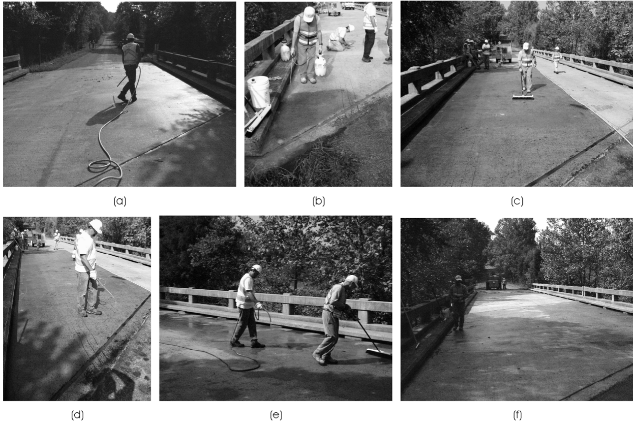
Figure 2. Application of TPS-II. (a) Bridge deck surface cleaned. (b) Inhibitor applied to surface. (c) Broom used to distribute product across surface. (d) Treated surface kept moist through periodic applications of water. (e) After a second treatment cycle, water used to rinse residue off treated surface. (f) Treatment complete.
